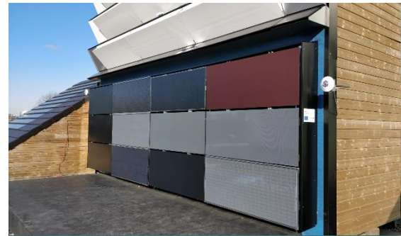
Figure 2: The outdoor colored and textured PV façade demonstrator installed at SolarBEAT, Eindhoven.
